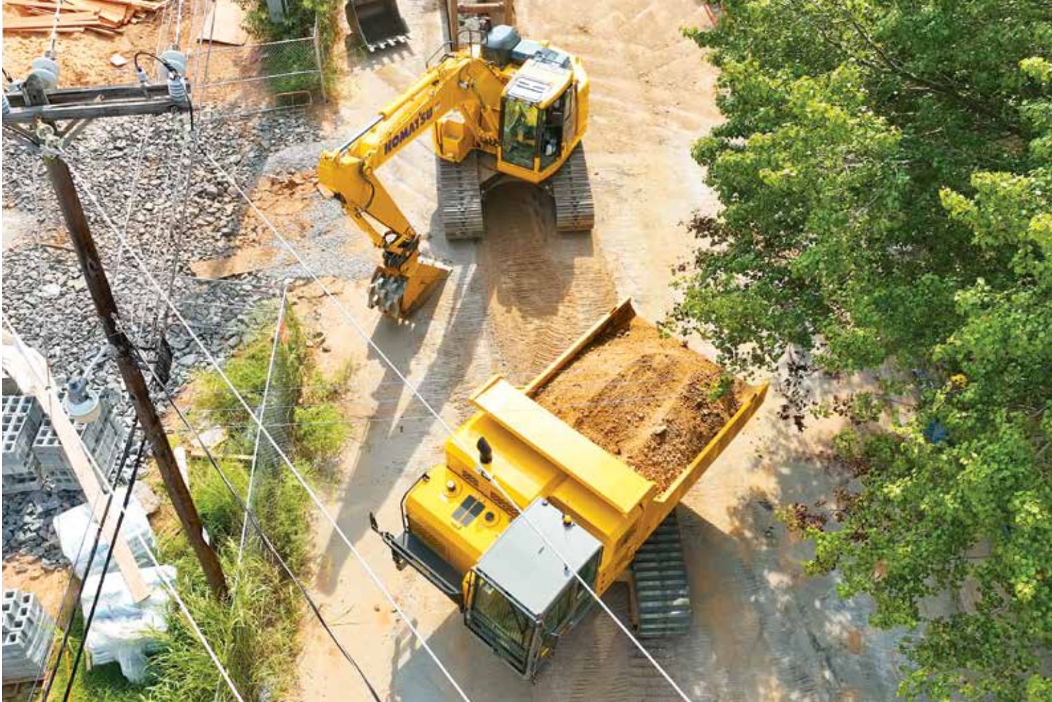
An operator rotates a Terramac RT14R crawler carrier 180 degrees to place material at the base of a Komatsu PC138USLC tight tail swing excavator.
