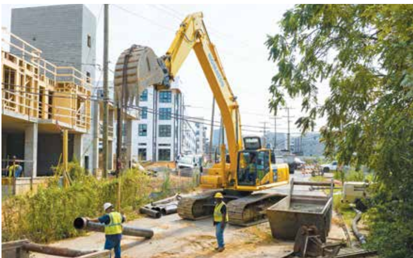
A crew moves a pipe into position with a Komatsu PC490LC-11 excavator.
